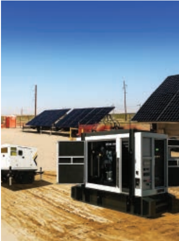
Power Rental & Energy Solutions
